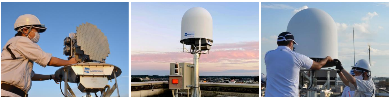
Installing an EAGLE radar in Yachimata City, Chiba Prefecture, for a field test
